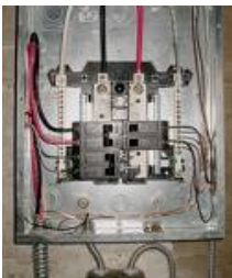
4 wires from meter...
